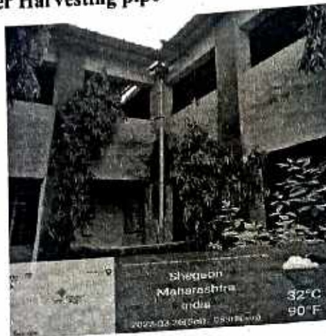
Photograph of Rain Water Harvesting pipe
