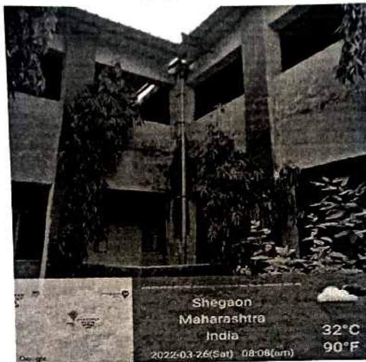
Photograph of Rain Water Harvesting Pipe:
